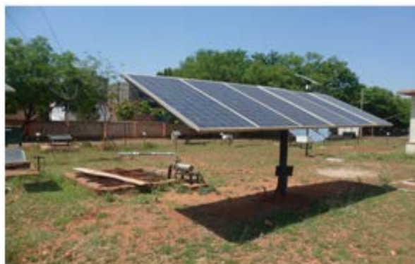
Fig. 1. Test system at Energy Park, BEC, Bagalkot.
